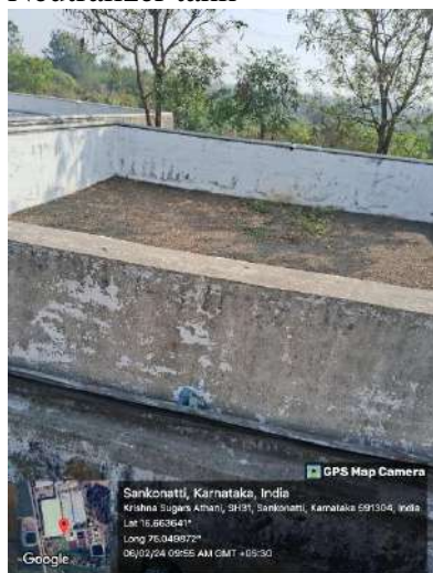
Sludge drying bed
