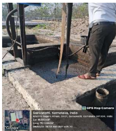
Photo: Oil & grease trap
